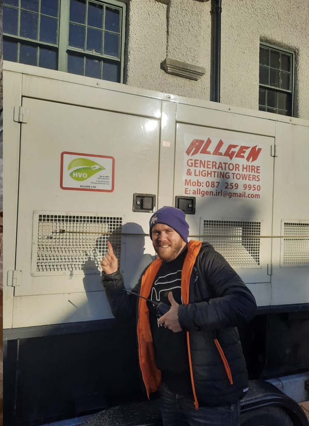
Bobby, from Locations with the generator running on HVO fuel.
